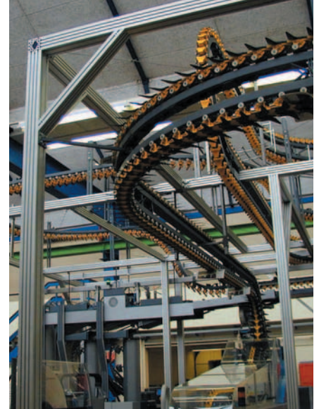
Newspaper handling system
